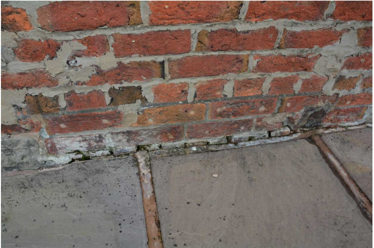
Repointing required to lower courses.
