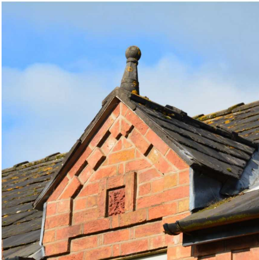
Cracked verge mortar.
