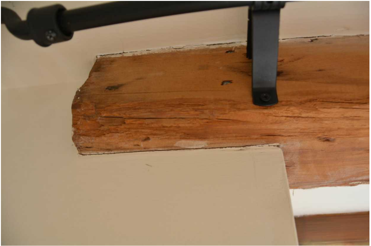
Softness noted to timber.
