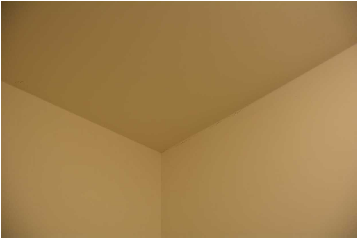
Cracking along plasterboard joints.
